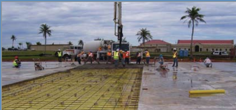
Contractors pour concrete for the foundation of a new 165,000 square foot base exchange building. Credit: U.S. Air Force photo
